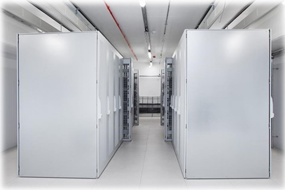
Colocation Cage Global Connect Datacenter Nydalén
